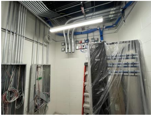
HS Data / Electrical Room
