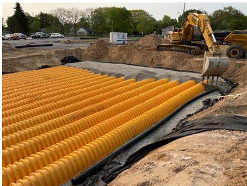
HS Staff Lot Water Detention System
