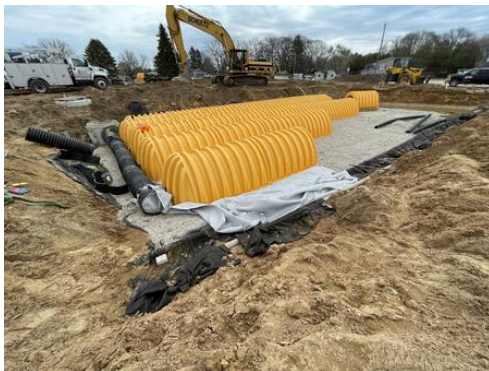
HS Staff Lot Water Detention System
